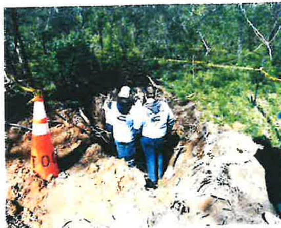
Soil Pit Station
